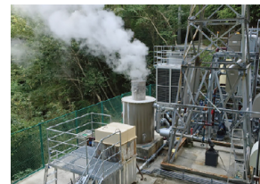
Binary cycle power generation (Shimoda Hot Springs)
