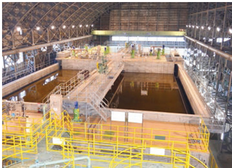
Motoyama AMD treatment facility at Toyoha Mine
