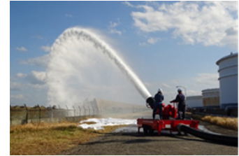
High-capacity foam water canon (Oita Refinery)
