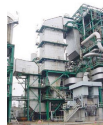
Flue gas denitrizer
