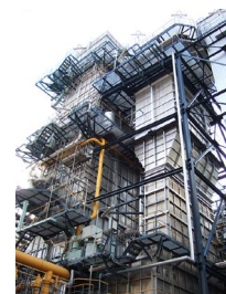
Flue gas desulfurizer
